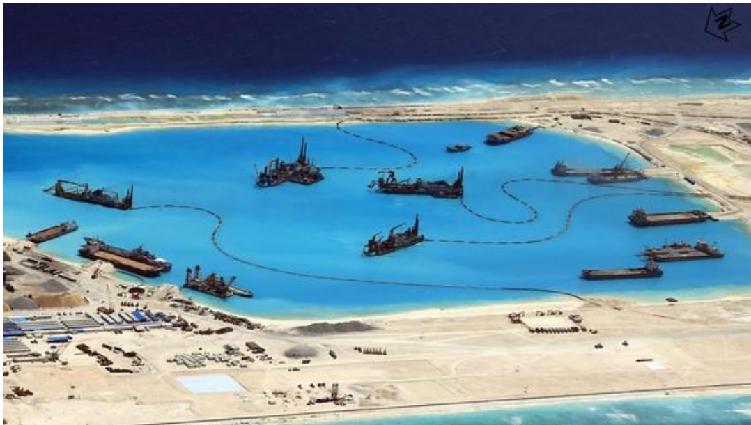
Chinese construction at Fiery Cross Reef in the disputed Spratly Islands in the South China Sea
